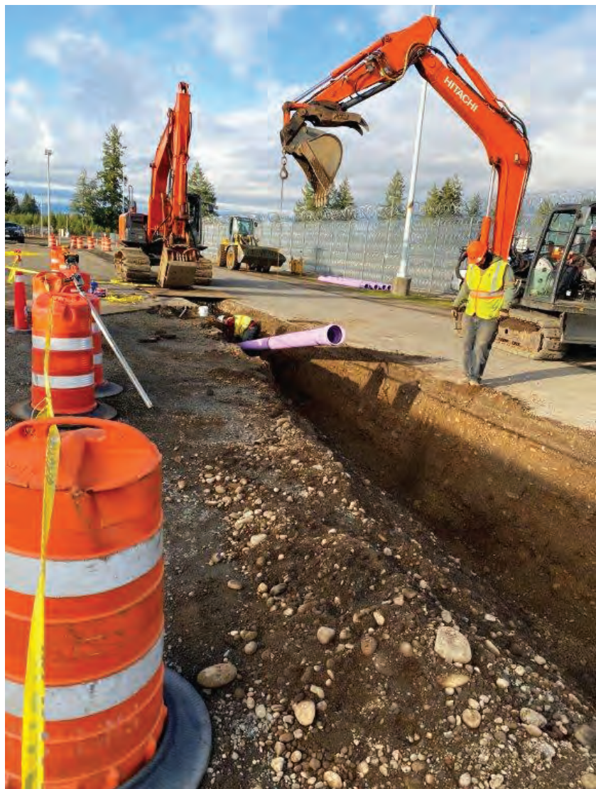
The Squaxin Island Tribe was a key partner in a project to send reclaimed water to Washington Corrections Center in Shelton. The project is expected to reduce the facility’s aquifer use. Photo: Squaxin Island Tribe
