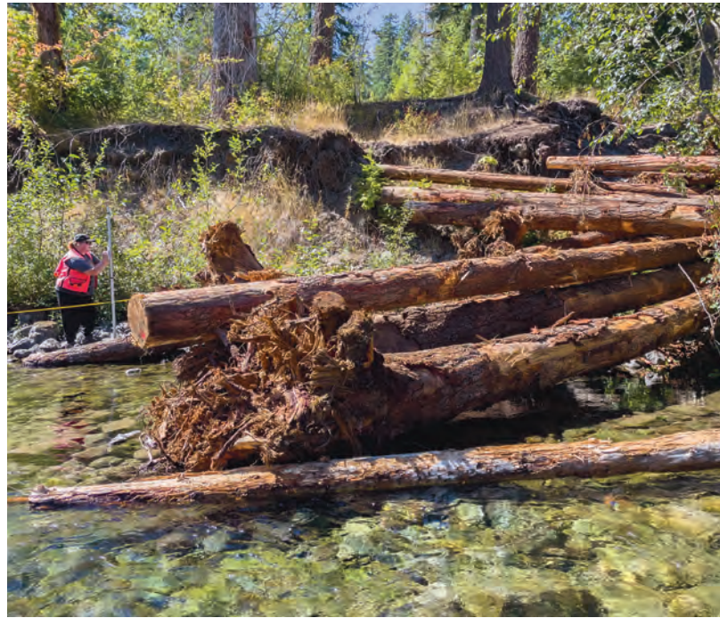
Above: Skokomish Tribe habitat biologist Lisa Belleveau takes measurements in the South Fork Skokomish River next to one of the recently installed logjams. Below: From left to right, Skokomish Tribe restoration planner Alex Papiez, Belleveau and Skokomish Tribe habitat program manager Alex Gouley evaluate the water level and new logjam in the South Fork Skokomish River. Photos: Tiffany Royal
