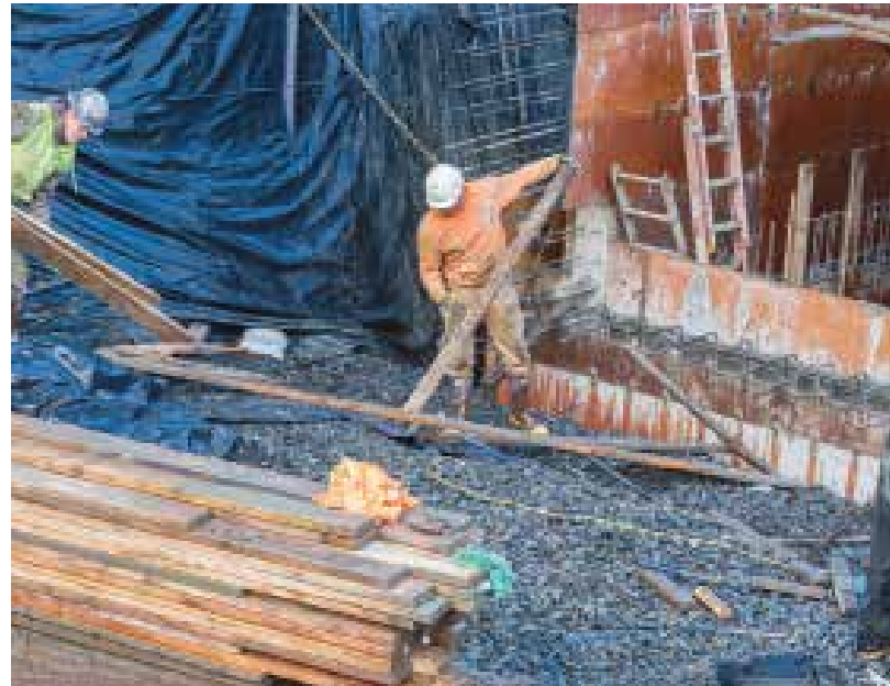
Construction workers with Chinook Enterprises work on the expansion of a raceway at the Bernie Kai-Kai Gobin Hatchery on the Tulalip Reservation. Photo: Richard Walker
